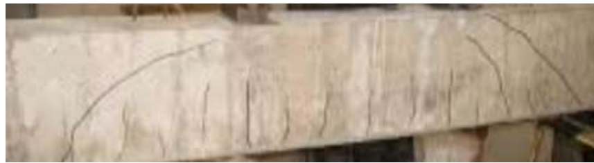
Fig. 2(a). Experimental Cracking Pattern in Control Beam
