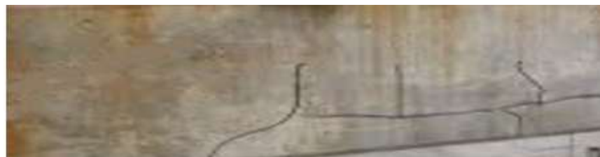
Fig. 2(b). Experimental Cracking pattern in 20% IOT Concrete
