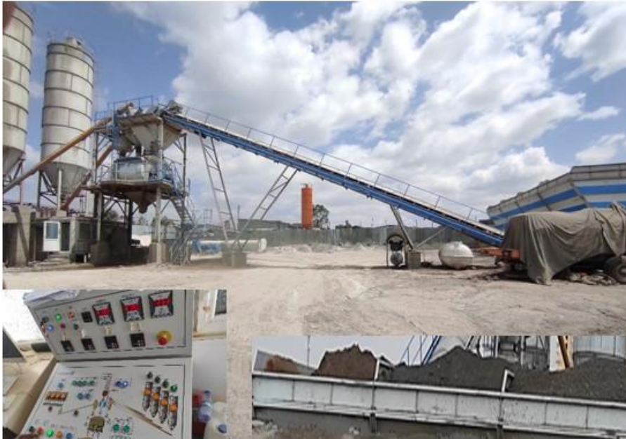
Figure 3: A typical stationary concrete batch plant located in Addis Ababa.
