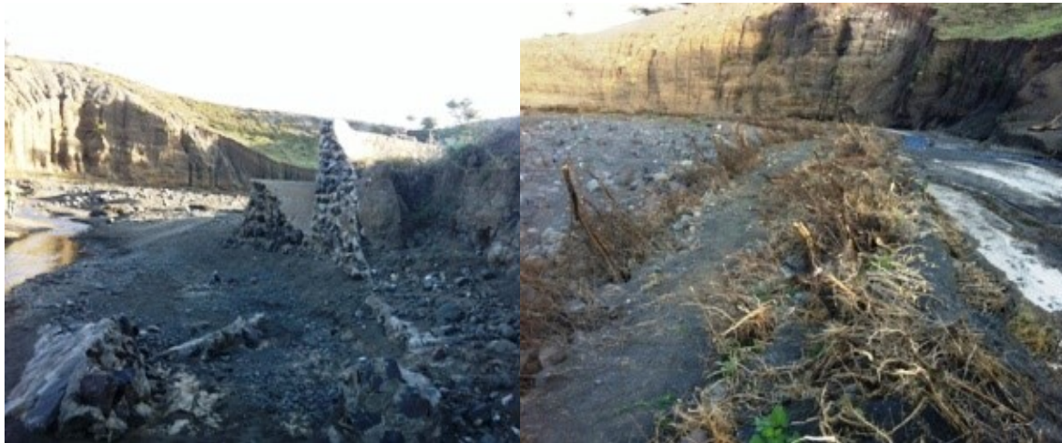
Broken diversion structure, Oda
